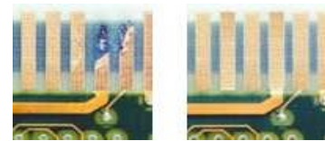
Before After Lands replaced with new dry film adhesive backed lands. Plated holes repaired with eyelets. Conductors repaired with Circuit Tracks.
